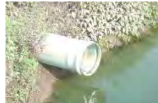
Edge of Field Drain Pipe
